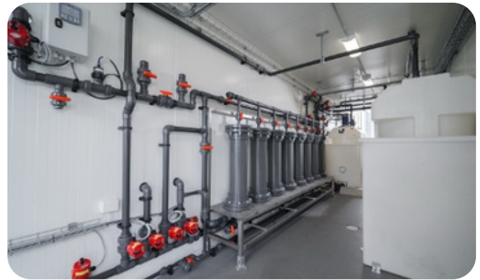
Figure 2: Picture of a 4D Scavenger unit designed for heavy metal removal from industrial wastewater. Picture shows the 4D Scavengers modules (8 pieces) as well as process piping and equipment.
